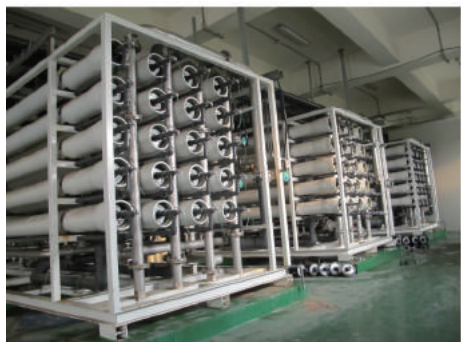
RO 逆滲透設備 Reverse Osmosis
