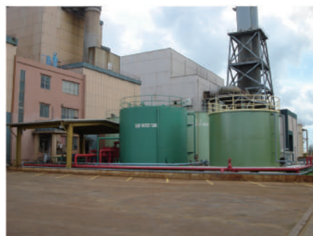
原水槽 Raw Water Tank
