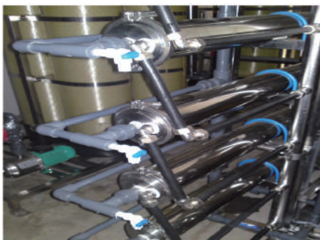
RO 設備 RO Equipment
