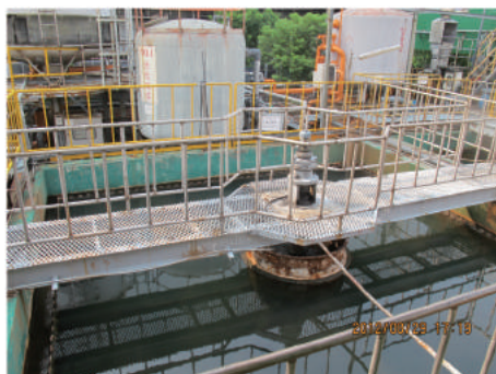
廢水池 Waste Water Tank
