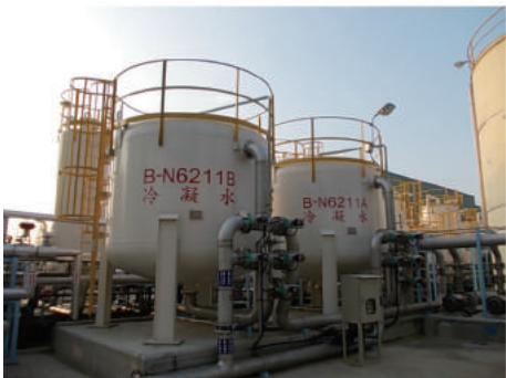
冷凝水設備 Cooling Water Equipment
