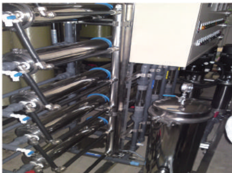
RO 設備 RO Equipment
