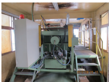
污泥脫水設備 Sludge Dewatering Equipment
