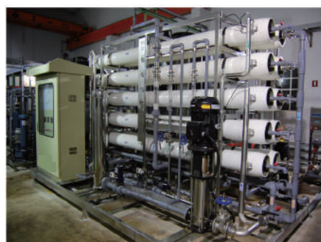
RO 逆滲透設備 Reverse Osmosis
