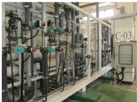
RO 逆滲透設備配管 Reverse Osmosis Pipes
