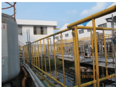
廢水池 Waste Water Tank
