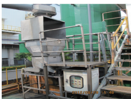
活性碳粉添加器 Powder Carbon Injection System
