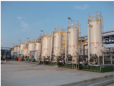
超純水設備 Ultra-pure Water Equipment
