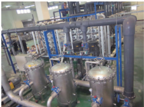
RO 前過濾設備 RO Pre-treatment Equipment
